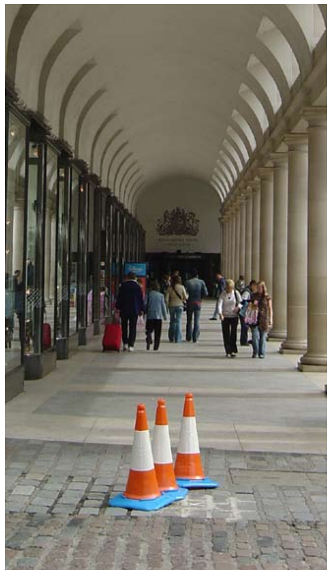
An example of the ongoing repairs to the setts in the Central Piazza.
